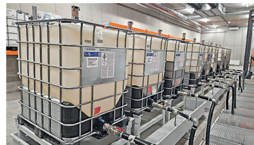
Neatly lined up reusable IBC containers supply Mayr Melnhof Holz's CLT plant in Leoben with Türmerleim's Elastan TLP adhesive
